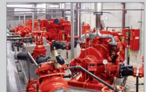
Horizontal Split Case Fire Pumps with diesel engines.
