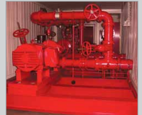
Completed housed unit.
